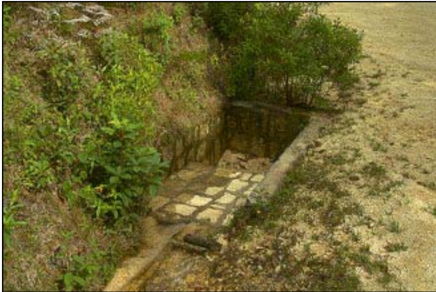
Photo 7.3 Use masonry, concrete, or metal inlet structures to control water in the ditch, direct the water into the cross-drain pipe, and prevent ditch down-cutting.
