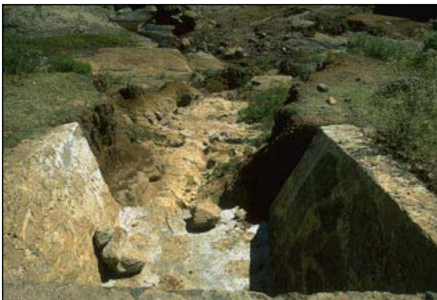
Photo 7.4 Add outlet protection and/or energy dissipators to prevent erosion and the formation of gullies.
