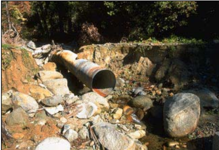
Photo 8.2 A culvert failure caused by insufficient flow capacity or inadequate pipe size to pass the debris (boulders) moving through the drainage.
