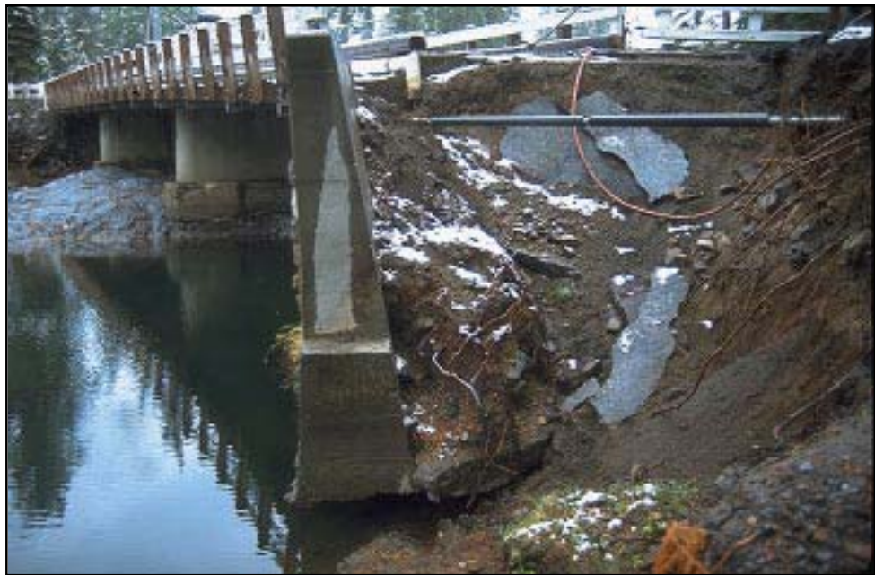
Photo 6.1 Scour behind a bridge abutment caused by insufficient channel and stream bank protection during a flood.
