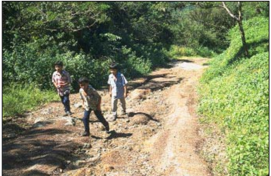
Photo 2.4 Adverse environmental impact from road surface erosion caused by steep road grades and insufficient cross-drains. This road is also difficult to maintain.
