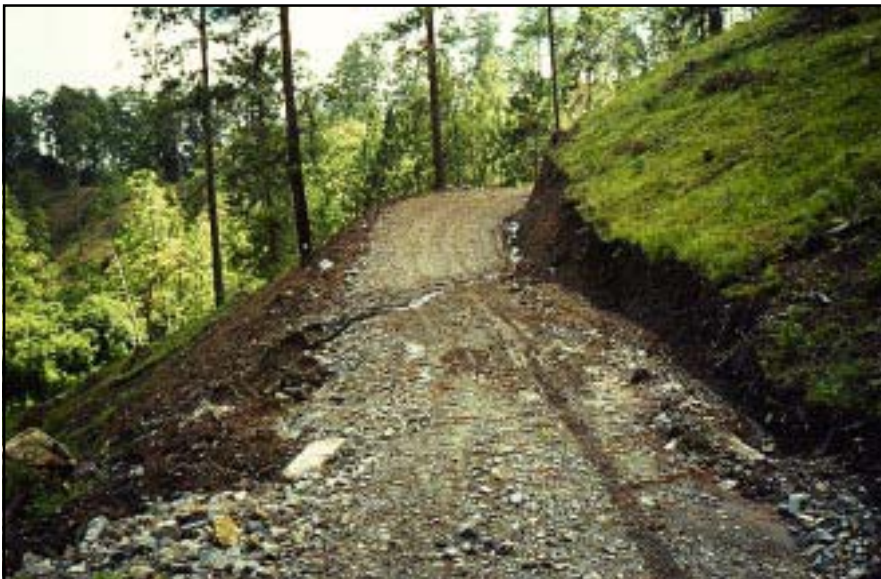
Photo 4.3 Avoid constructing roads with steep grades or on steep side slopes. It is difficult to control drainage with steep road grades.
