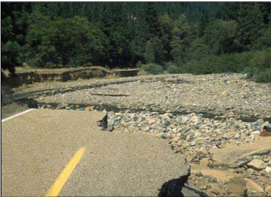
Photo 3.3 A poorly located road, in the hazardous flood plain area of a river, that has washed out during a major storm event.
