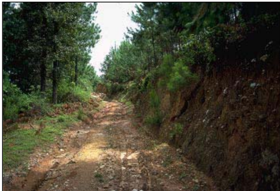
Photo 12.1 A rutting road caused either by soft subgrade soil or inadequate road drainage (or both).
