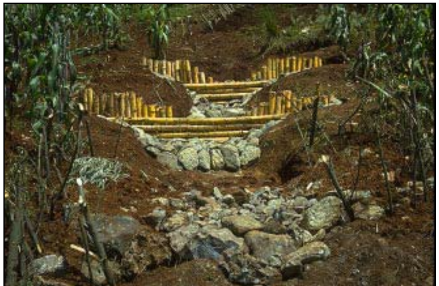
Photo 14.4 Construct debris retention and gully control structures with a notched weir to keep flow over the middle of the structure, add scour protection at the outlet of each structure, and key the structures into the firm soil banks.
