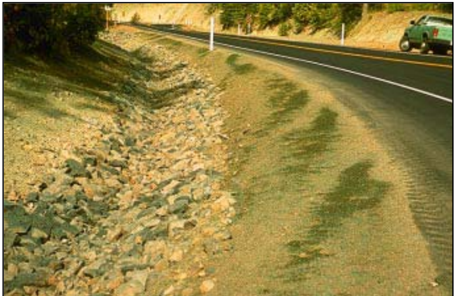
Photo 3.5 Maintain roads and drainage features to withstand major storm events with minimum erosion, such as with armored ditches that are kept clean.
