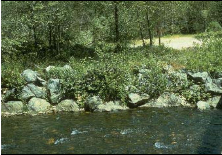
Photo 6.2 Riprap used for stream bank slope protection to prevent scour at the entrance of a structure. Note the use of willows for additional “biotechnical” root strength.
