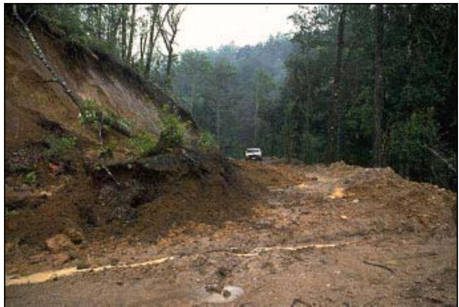
Photo 1.3 A problematic road because of roadcut failures. Instability problems cause road user delays, and high maintenance or repair costs.
