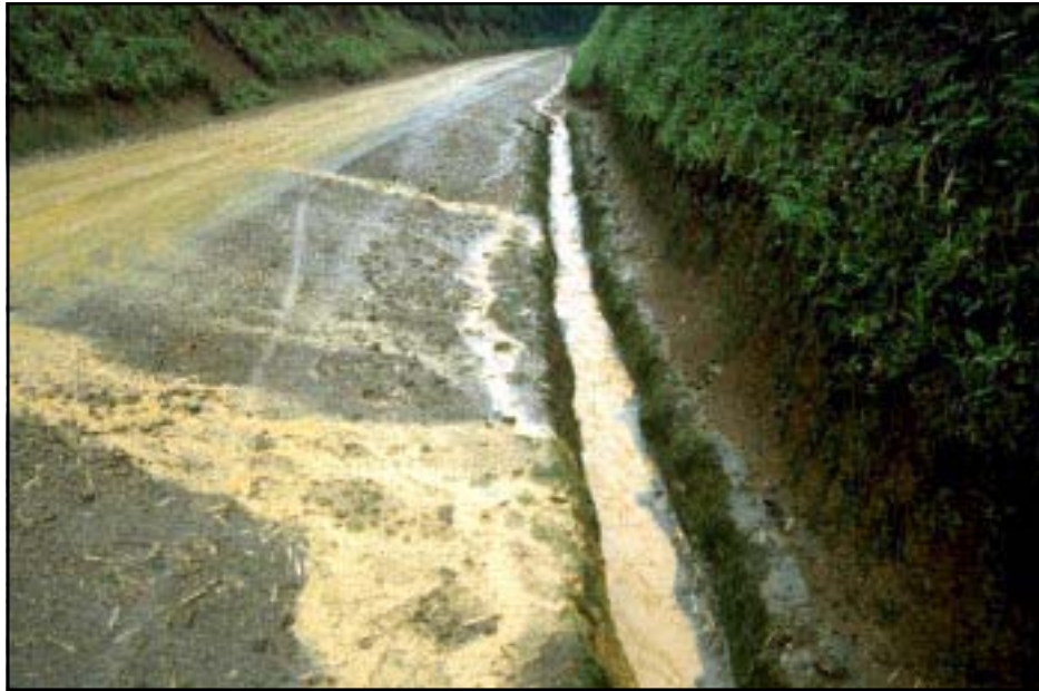
Photo 7.6 Armor ditches with vegetation, rock, masonry, or concrete to resist ditch erosion and carry the water to a stable exit point.
