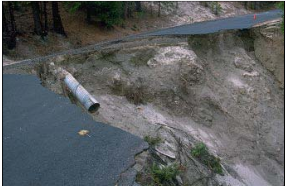
Photo 11.10 A road fill failure in steep terrain which now needs either a retaining structure or a large road cut around the failure.
